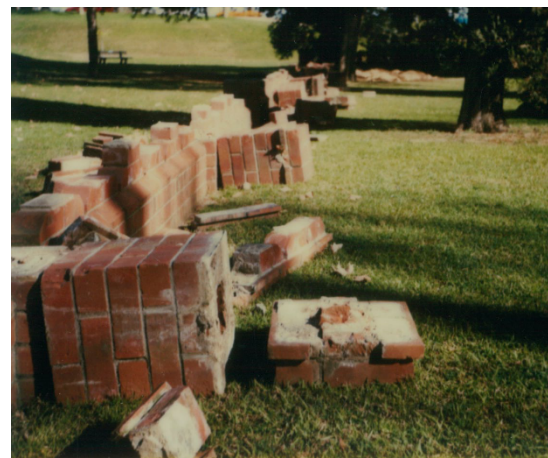
Figure 24. The damage to the wall was substantial. Source: PWMGT
