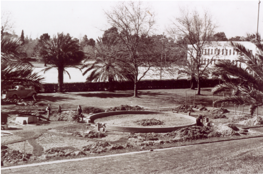
Figure 9. The foundations for the wall and the brickwork around the raised platform being laid.
